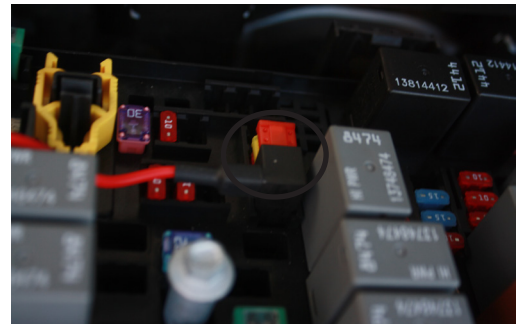
Figure 3: JL Power Connection
